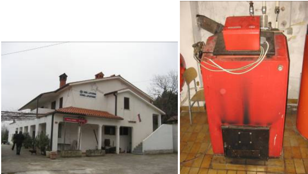
Figure 3: Truške Inn and the boiler with the burner currently used
