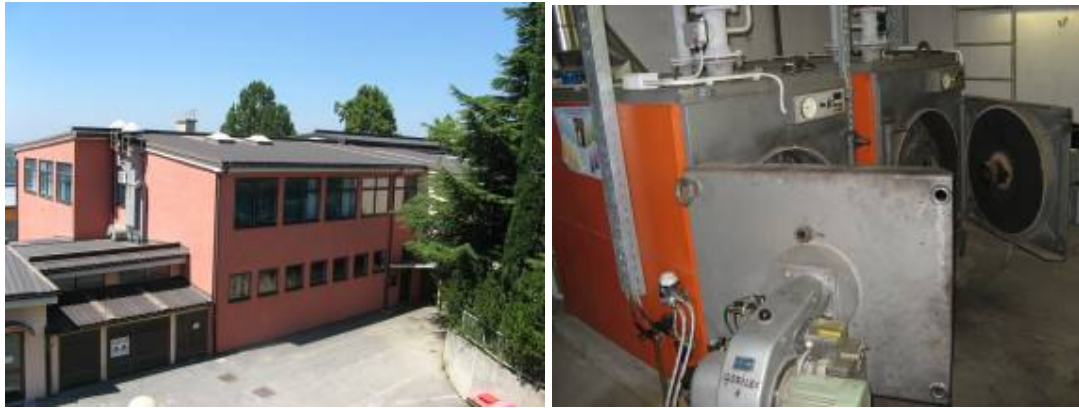
Figure 3: ŠPS and the boilers currently used
